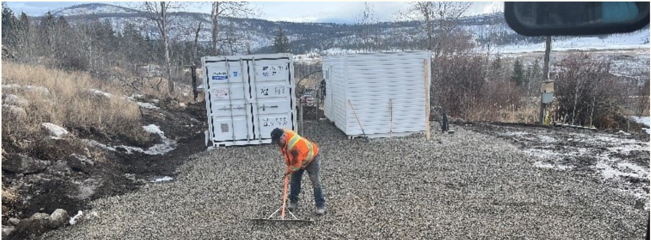
Levelling the ground at the Hanceville site, with the TNG interim hatchery-in-a-box (2 seacans) in the background (February 2023).
